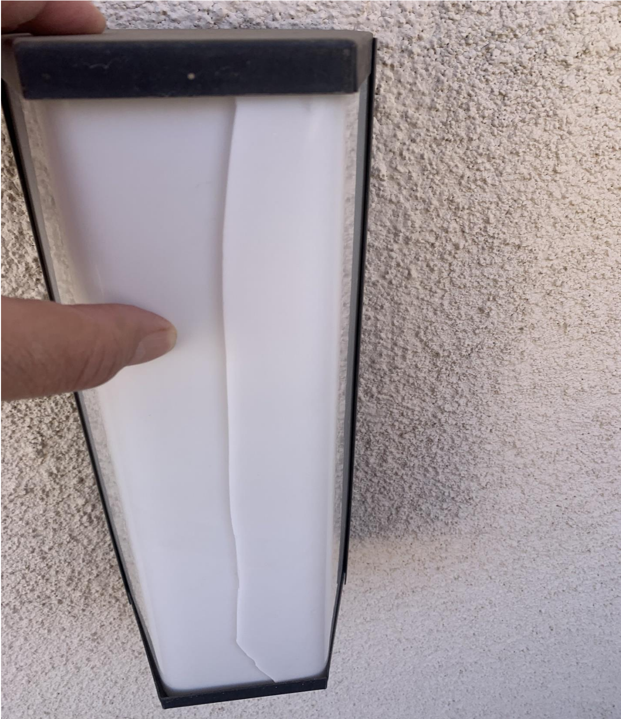
Cracked Light west side of 313 (courtyard side)
