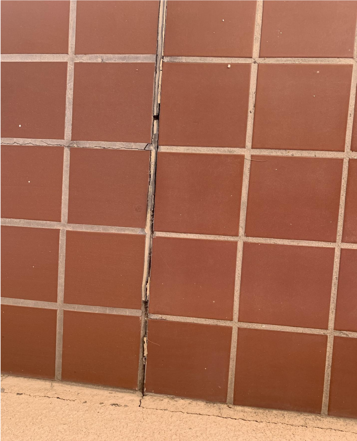
Loose tile near p7 courtyard side
