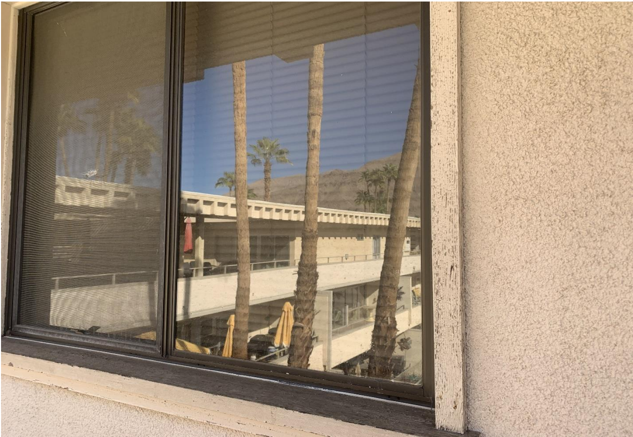
3 rd floor near 312 courtyard side, match paint near downspout and windowsill.
