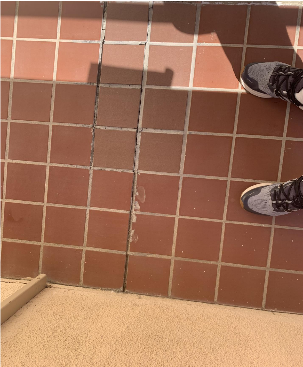
Loose tile near P8 courtyard side.
