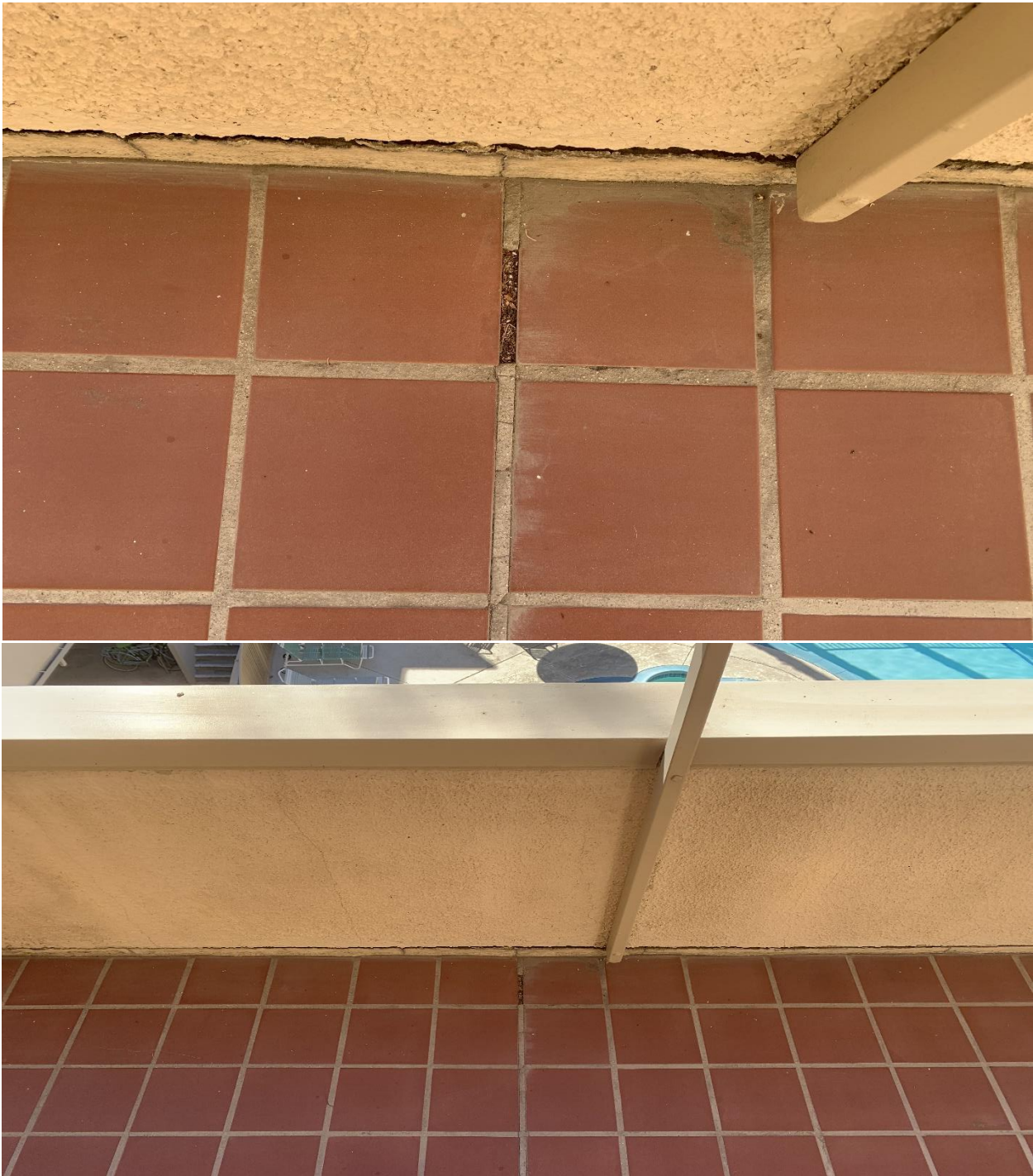
Loose tile near p10 courtside
