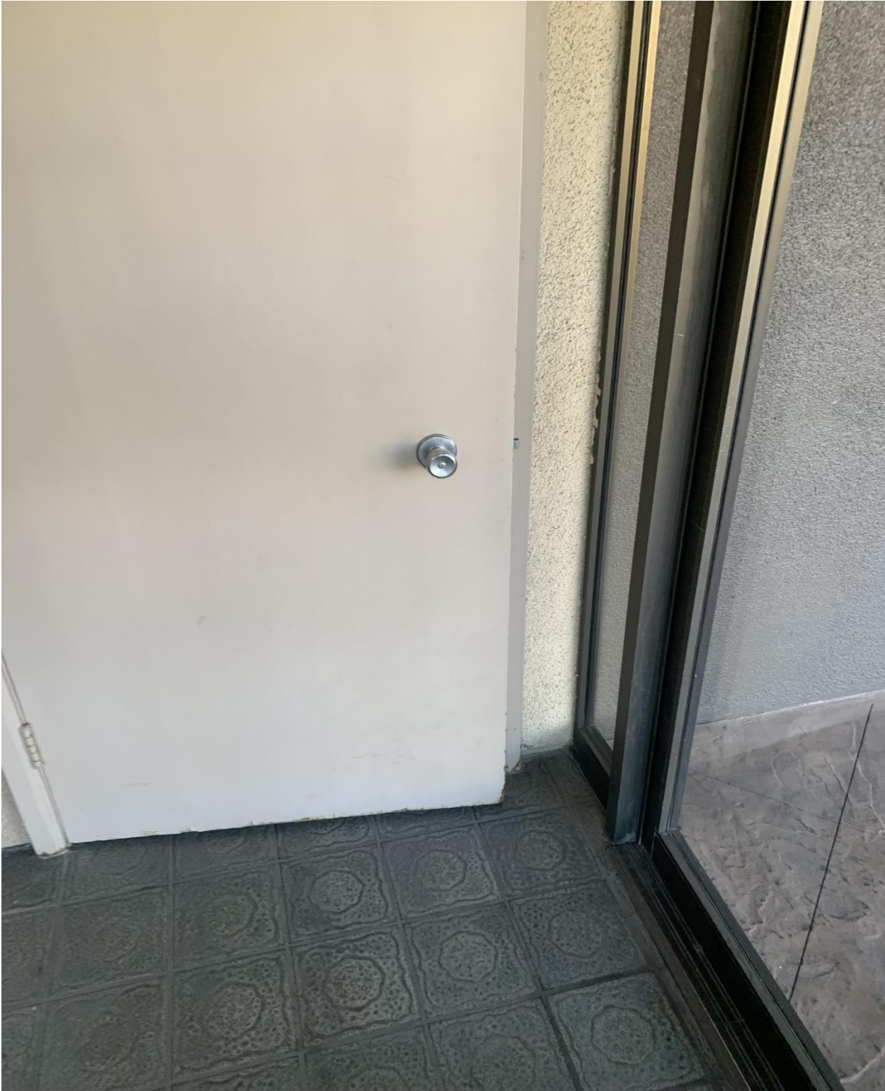
First floor northwest fix non-closing trash room door
