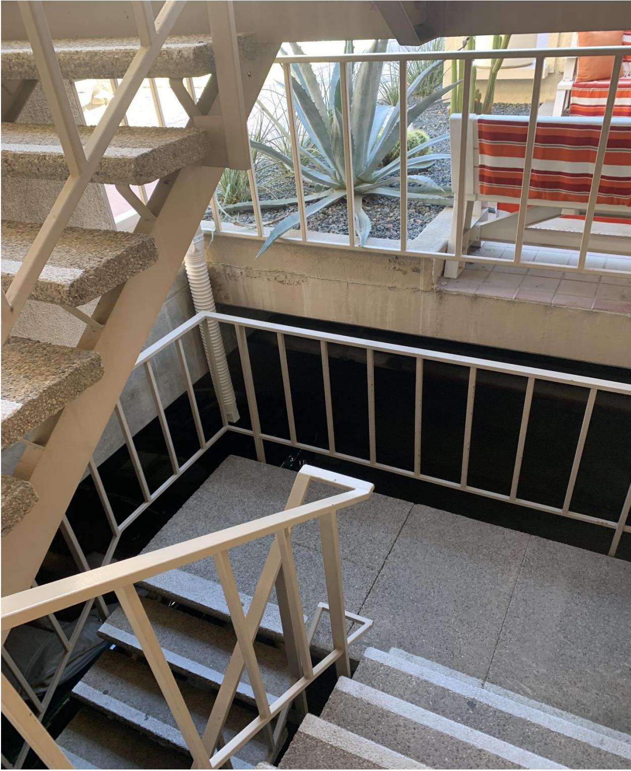
Paint corner of stairway near 101.... Maybe all of the stairway rails need attention.
